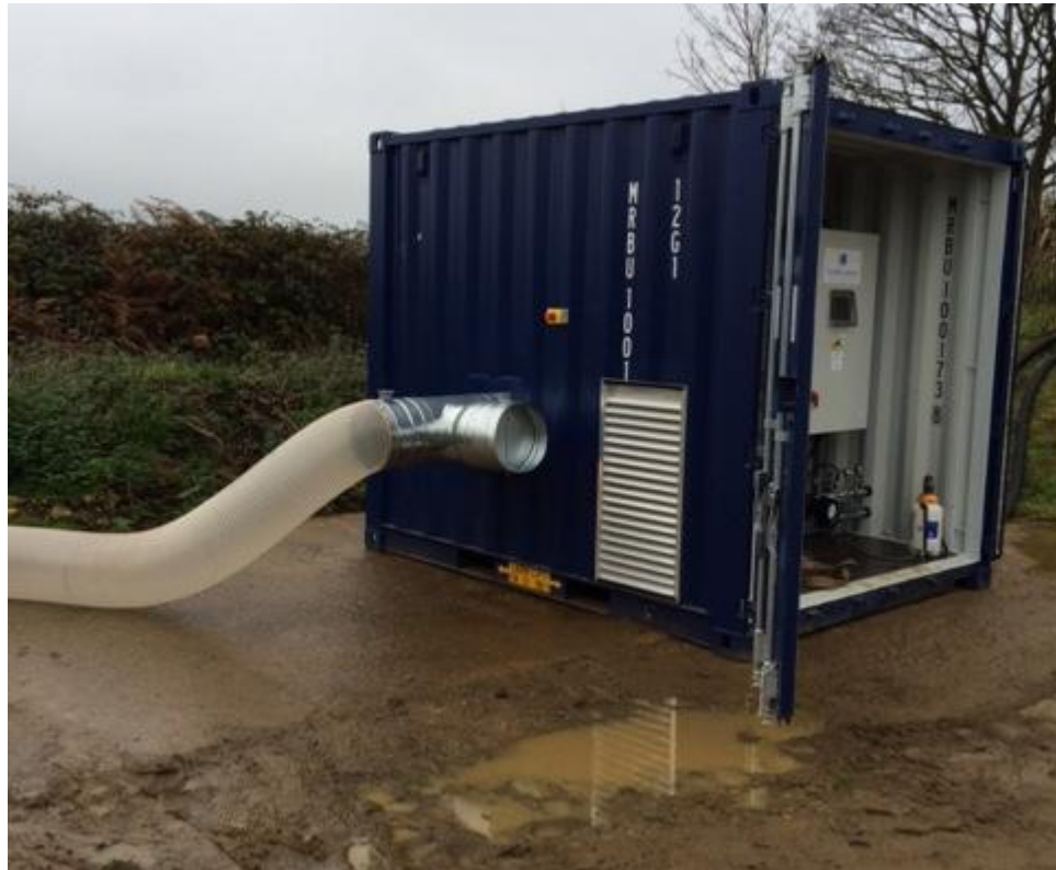
Heat transfer unit at Docking 2 with hot air piping attached.
