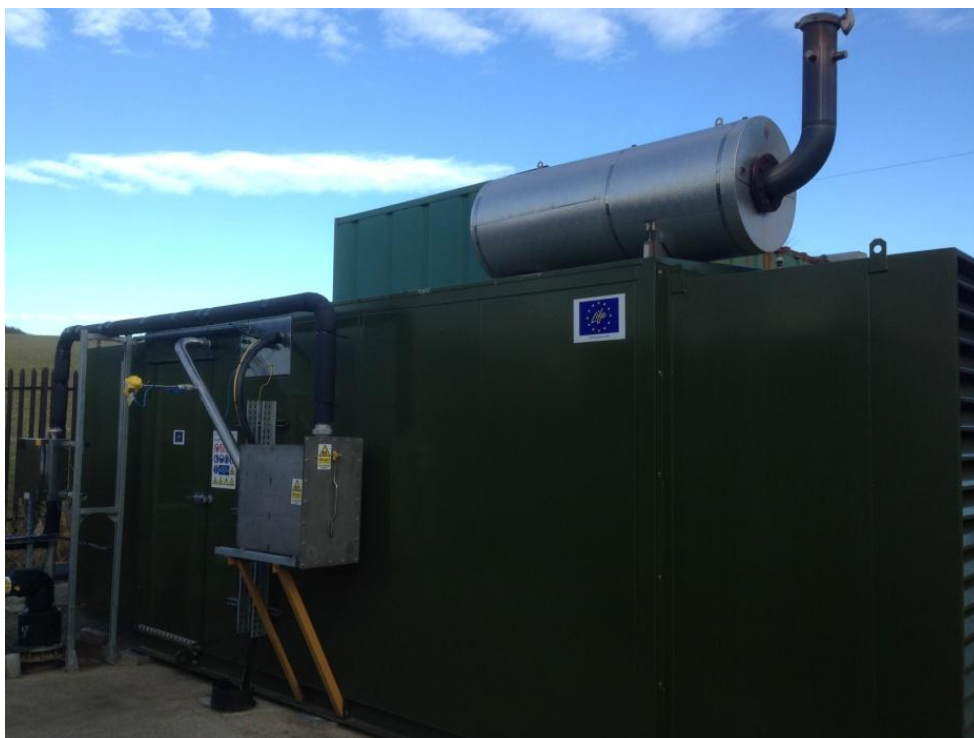
A small-scale spark ignition engine as installed at one of our ACUMEN demonstration sites in the UK.
