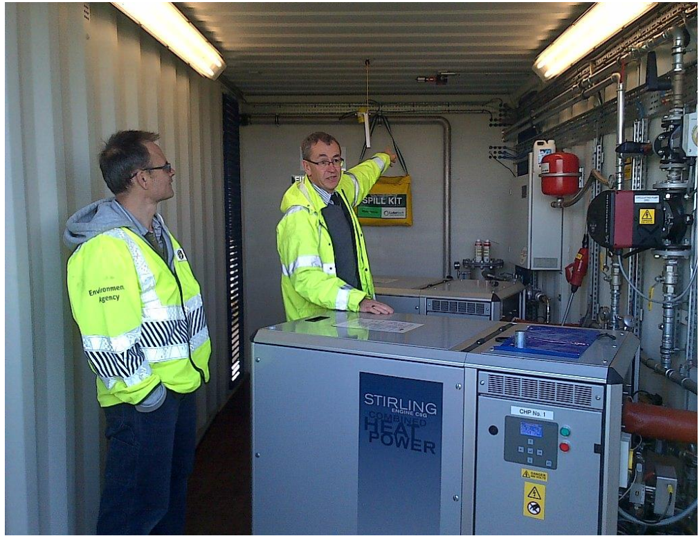
Two external combustion Stirling engines in use at one of our ACUMEN demonstration sites in the UK.
