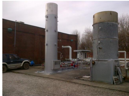
The gas management compound at Otterspool
