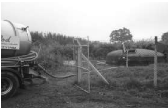
Routine desludging of iron precipitation from header tank
