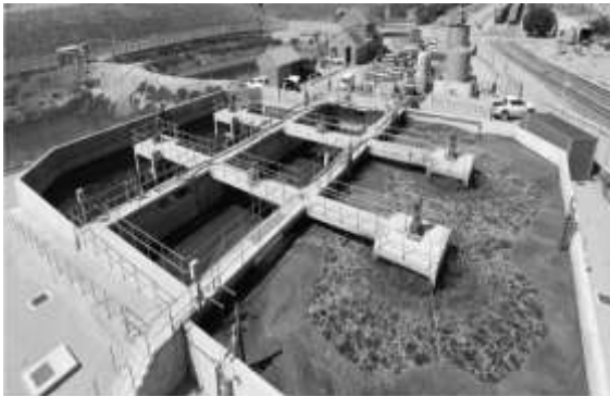
Vissershok LTP, Cape Town, commissioned 2011
